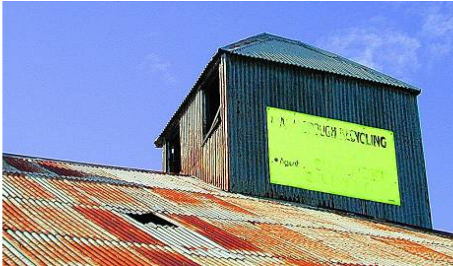
“RUSTY ROOF” ROB CROSS
